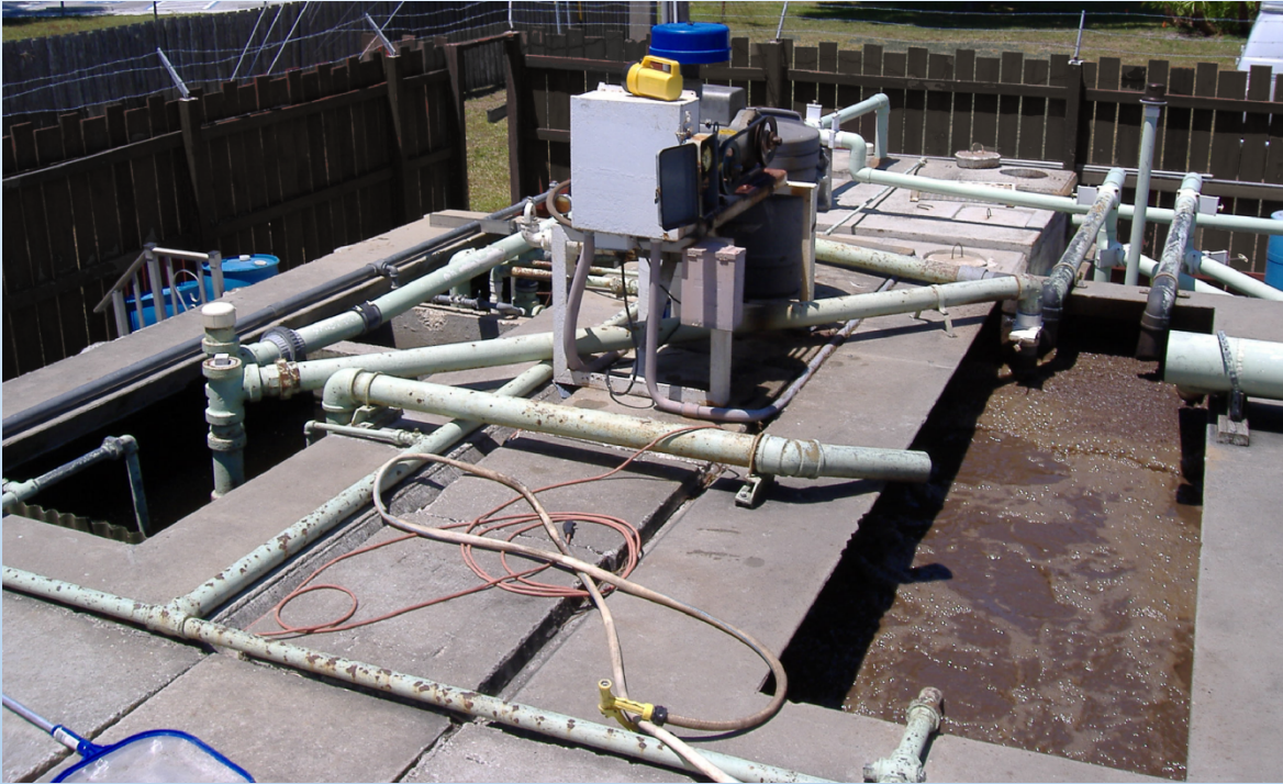
Conventional Activated Sludge Category of Treatment
