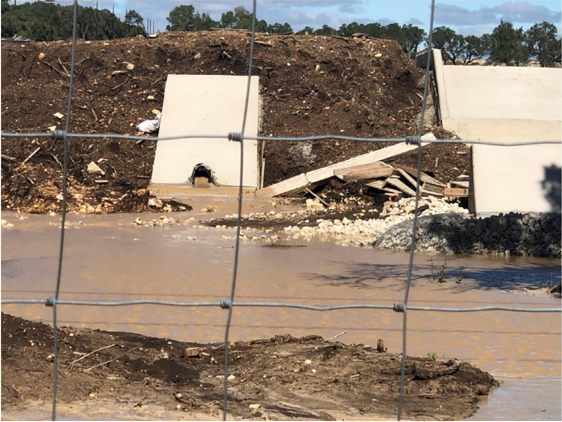
Figure 1 October 25, 2019 photograph of storm water containing sediment exiting Detention Basin D on Development Property
