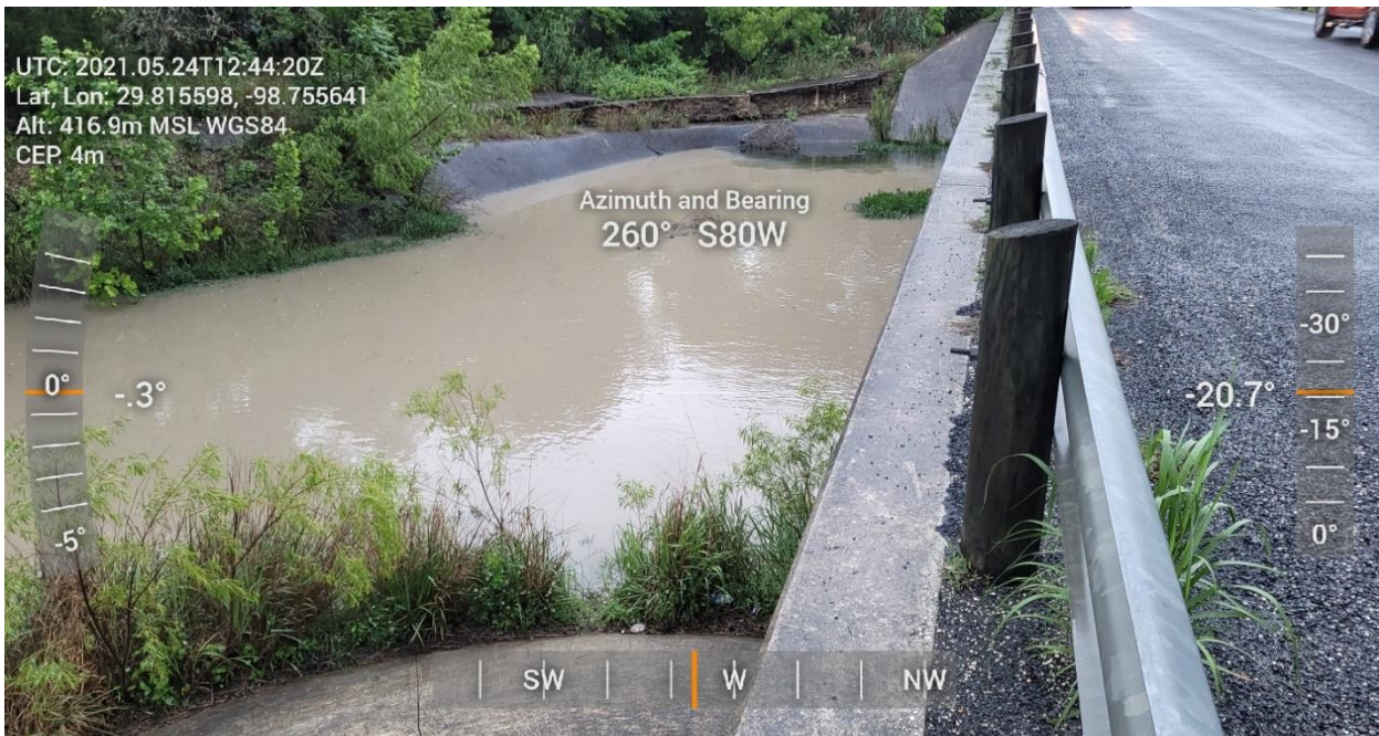
South side of Ranger Creek Road Bridge Over Cibolo Creek, May 24, 2021, 7:44 AM CDT
