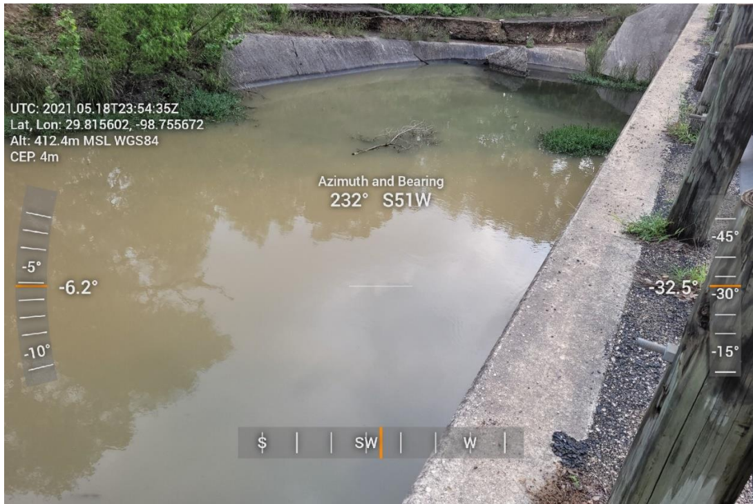
South side of Ranger Creek Road Bridge Over Cibolo Creek, May 18, 2021, 6:54 PM CDT
