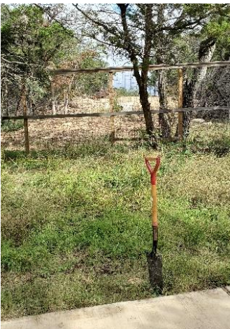
Figure 25: Culvert Site showing sediment deposition from the abutting property.
