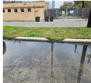
Figure 15: Silt removal is required to allow stormwater to enter the turf area.
