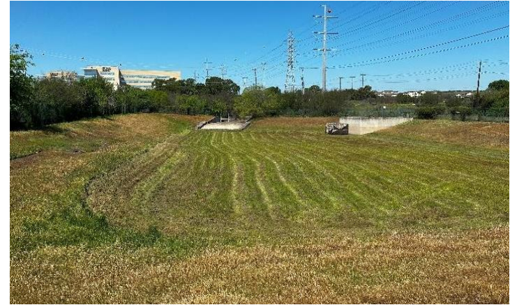
Figure 18: Sand filtration system properly maintained; no standing water, tree seedlings or debris. The turf height is also good.
