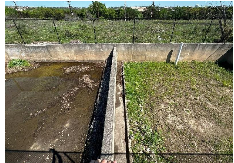
Figure 19: Standing water indicates maintenance required for proper filtration which would include sediment removal.
