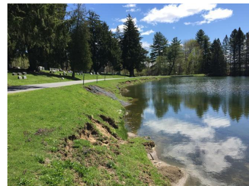
Figure 14 : Mowing to the edge causes erosion, bank failure and silt filling the lake.
