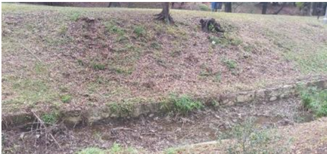
Figure 5: Slopes present a challenge; this vegetation has been cut too short increasing soil erosion and allowing weeds to grow.
