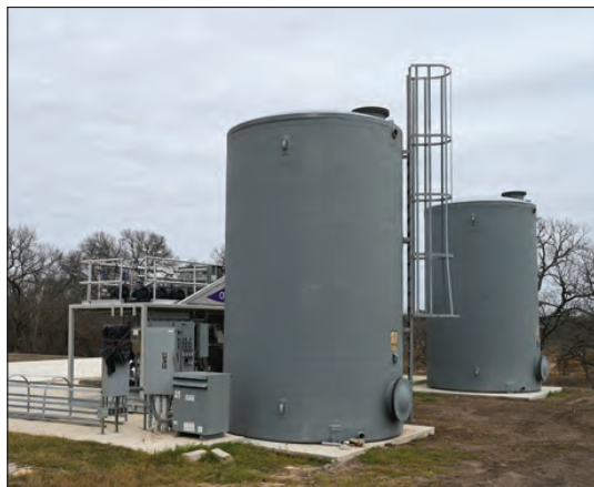
The water treatment facility installed at the development. This facility from a Taylor company will treat wastewater and allow the treated effluent to be reused onsite.
