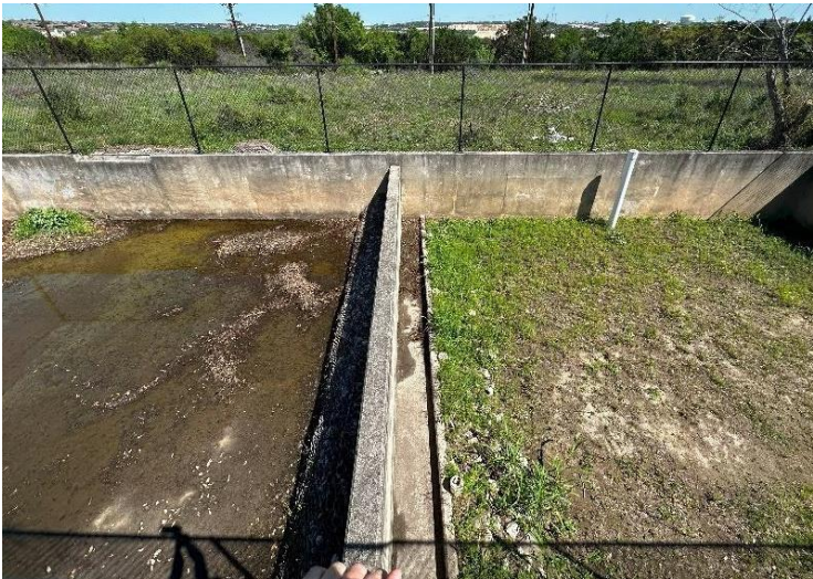
Figure 19: Standing water indicates maintenance required for proper filtration which would include sediment removal.
