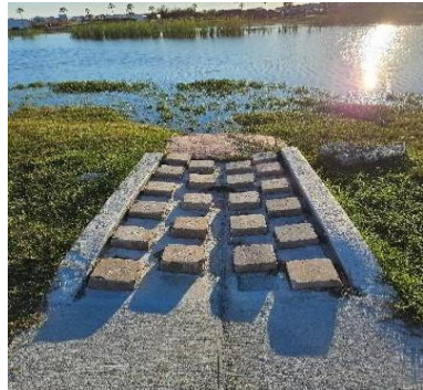
Figure 16: This feature directs and slows stormwater while preventing erosion.
