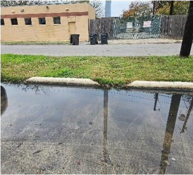
Figure 15: Silt removal is required to allow stormwater to enter the turf area.
