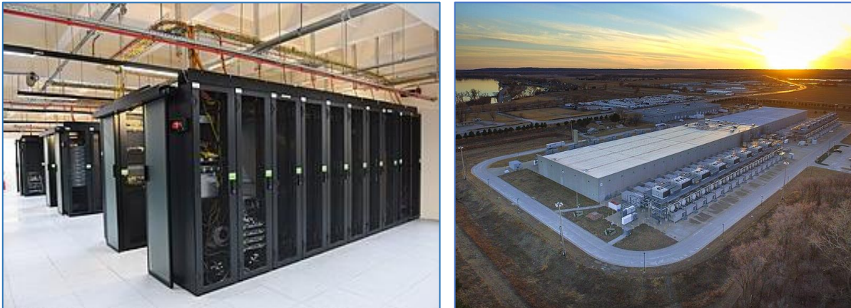
Figure 1. A view of the inside [4] and outside [5] of a data center, supplied by Wikimedia Commons.
