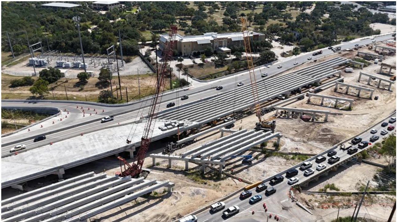
Fig. 4: TxDOT’s Oak Hill Parkway project has destroyed area flora, decimated animal habitat, and disrupted driver commutes for several years now. (image source: TxDOT)
